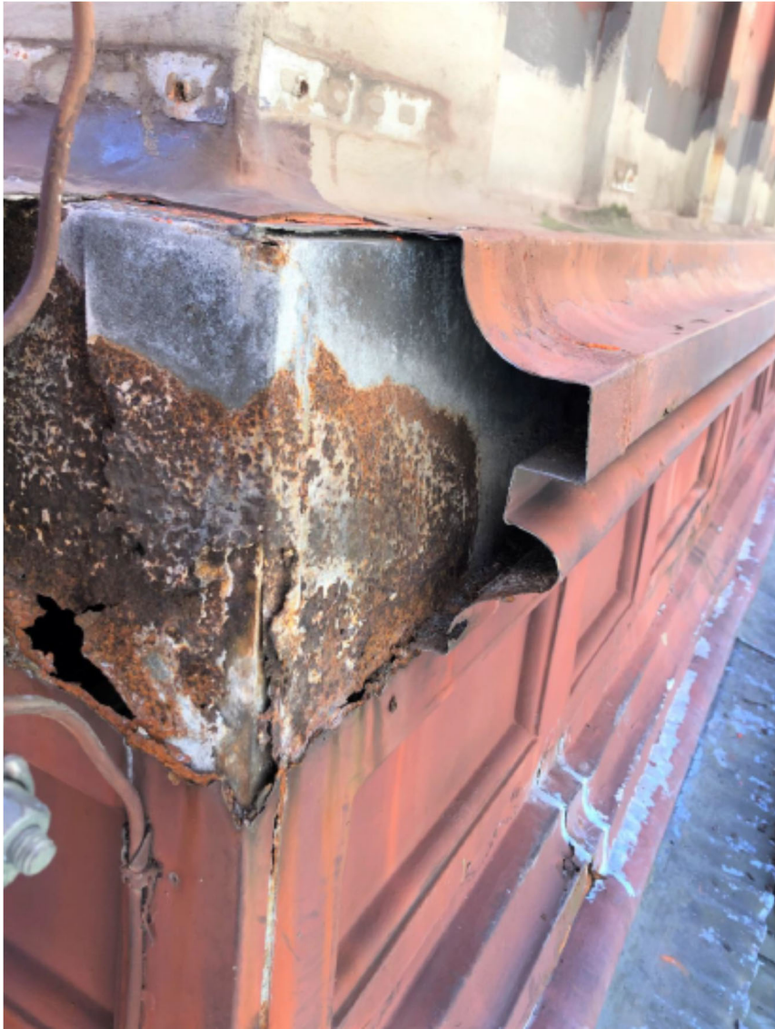
Figure 7. Dome Lantern, showing the deteriorated condition of the original galvanized steel sheet.
