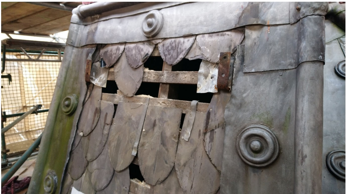
Figure 2. Deterioration to turret.
