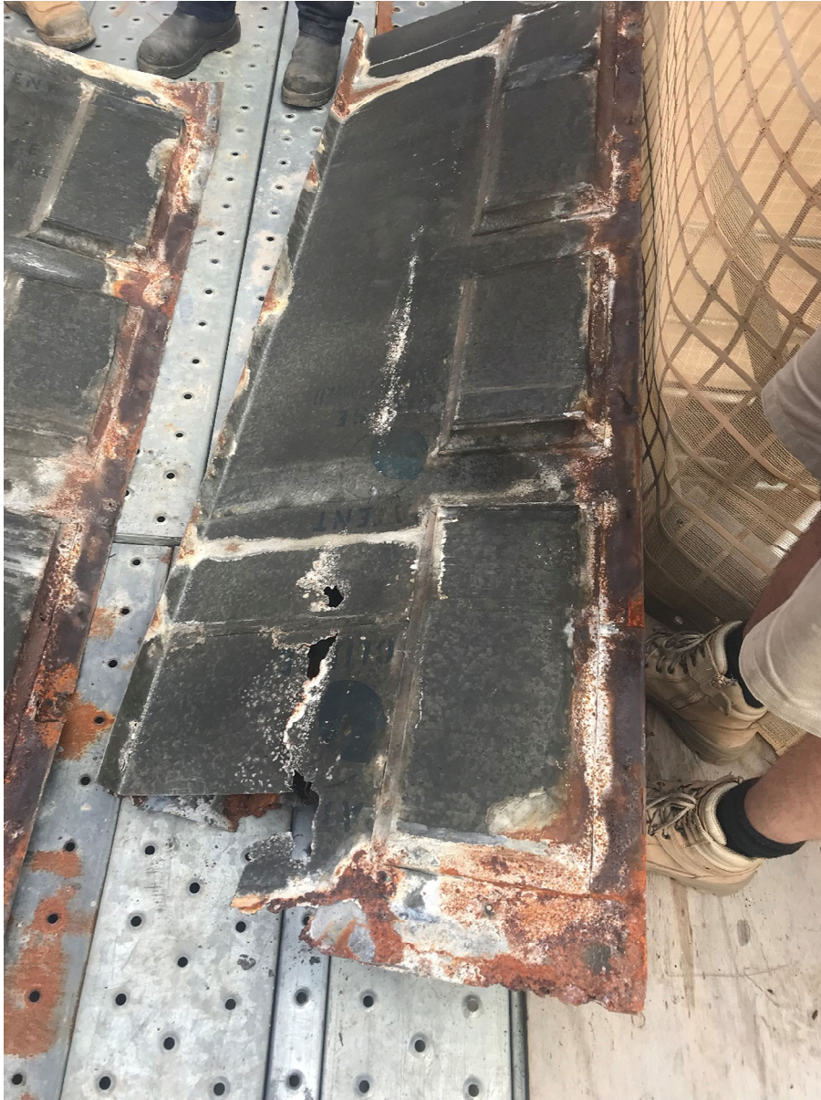
Figure 8. Dome Lantern, interior face of a portion of the removed original architrave panels with visible corrosion.
